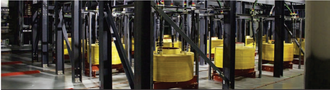
The Duke Energy Electrical Grid Research Innovation and Development center (eGRID) at Clemson can simulate the electrical grid of any country in the world to test how cities would manage cyberattacks to power infrastructure
